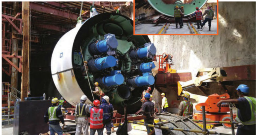
Yu Sin personnel lowering and bolting together the tunnel boring machine front body in preparation for a slide.
