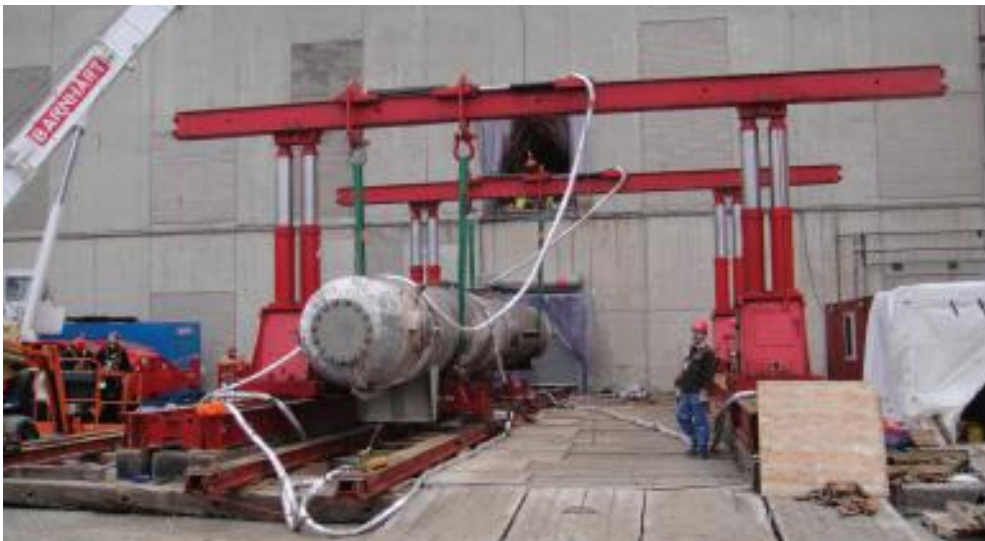
Barnhart Crane & Rigging used a Lift Systems gantry, slide track and 50-ton rough terrain crane to remove and replace three nuclear feedwater heaters
