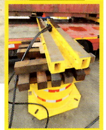
The HT300 heavy track skidding system using HS3014 hydraulic cylinders (insert) to move a container on skid tracks levelled by support stands and Ekki timber blocks.
